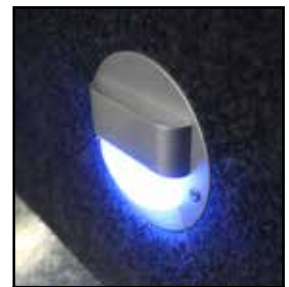
Low level interior lighting
